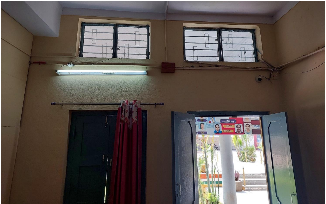
Figure 11- T5 & T8 tube lights with Electromagnetic choke
