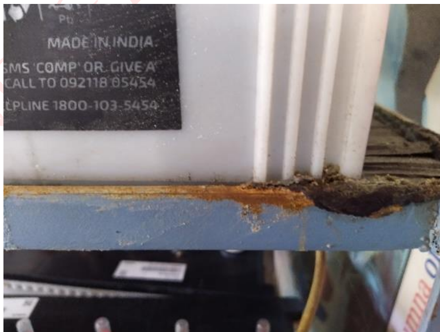
Figure 13 - Galvanic reaction causing damage to battery life.
